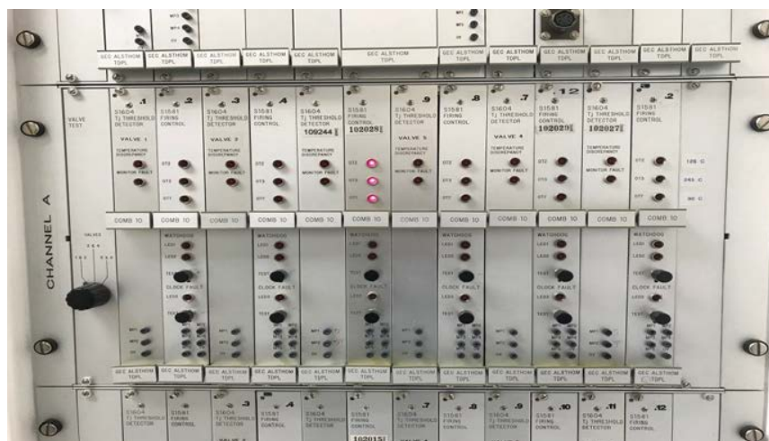
Figure 4.7. Mysterious fault in the TA&FC panel.
