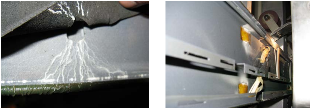
Figure 3.11. Damages caused by electrical tracking and partial discharge activities inside the LG channel.
