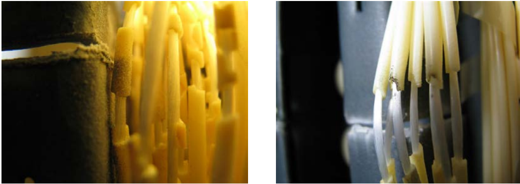
Figure 3.10(b). Severely deteriorated LG insulation jacket at Dorsey.
