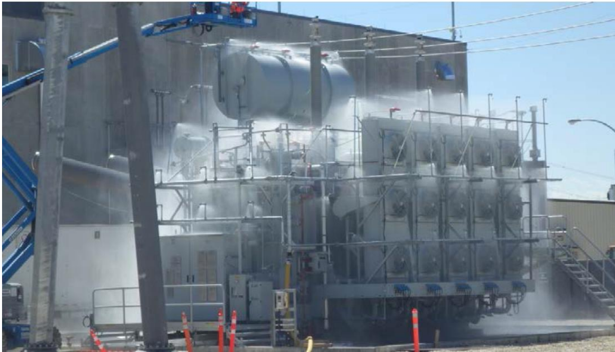
Photo 1: Riel Converter Station, spare transformer deluge testing
