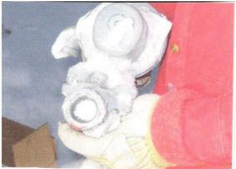
Figure 4.1 – Hydrates plugging a pressure regulator
