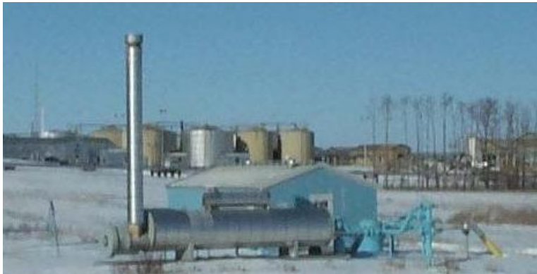
Figure 4.4 – Indirect line heater
