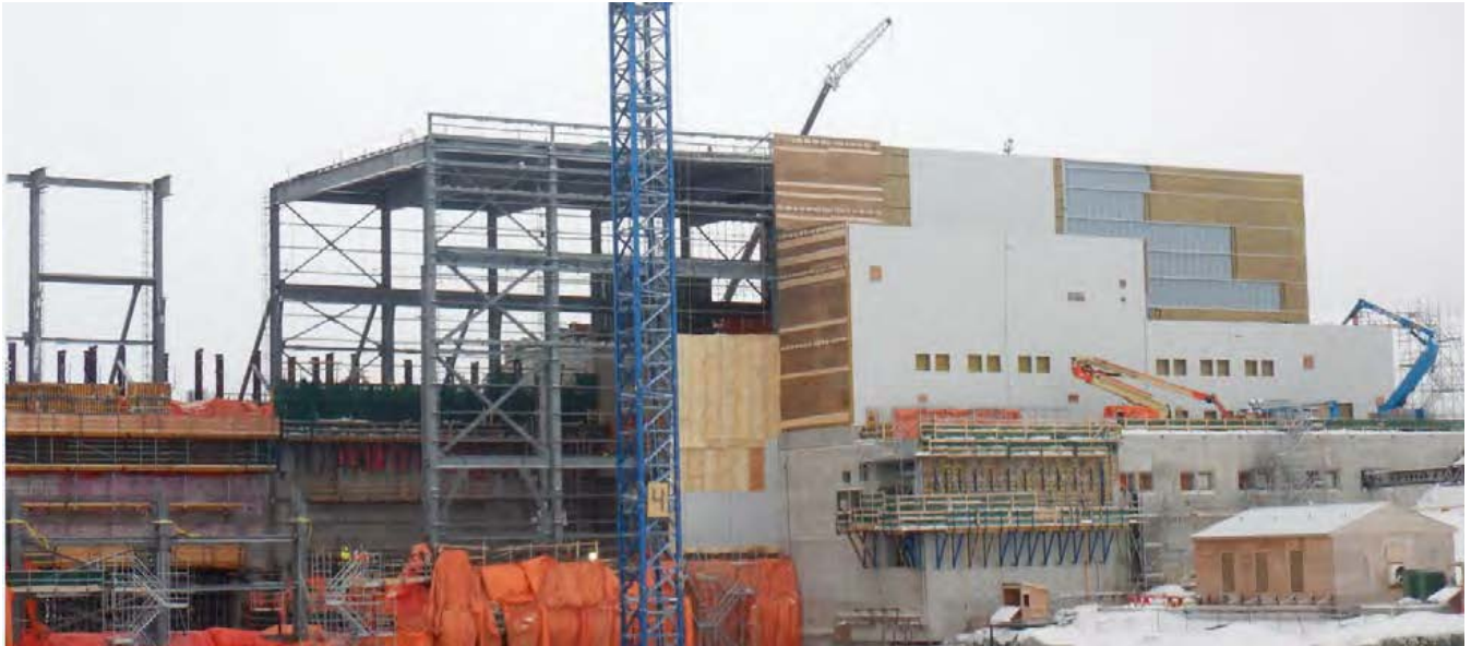
View of service bay and PH unit 1 looking upstream
