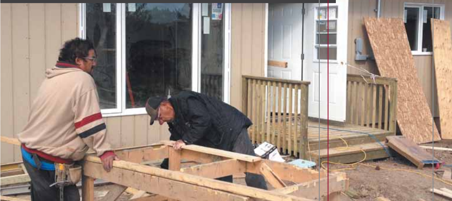
One of ten new homes being built in Sandy Lake First Nation, Ontario, where there are 154 applicants waiting for housing.
