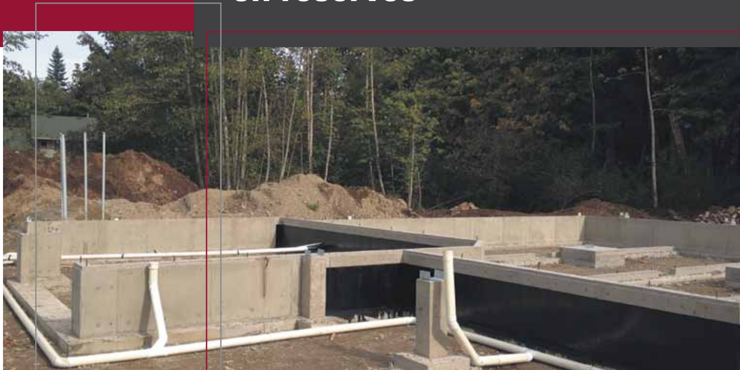
Housing construction in We Wai Kai First Nation in British Columbia is inspected by city inspectors.
