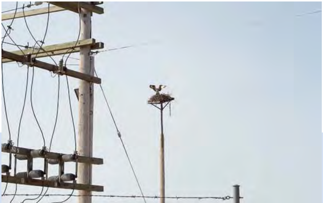
Osprey nest on platform located outside of substation.
