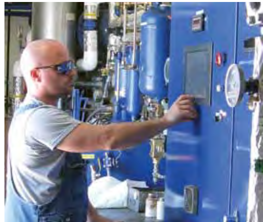
Control panel in PCBX rig used for decontamination of oil.
