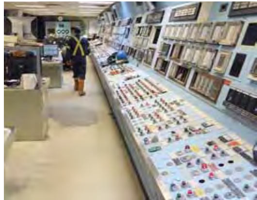
Tolko's Steam and Recover control room where monitoring of the burn test occurred.
