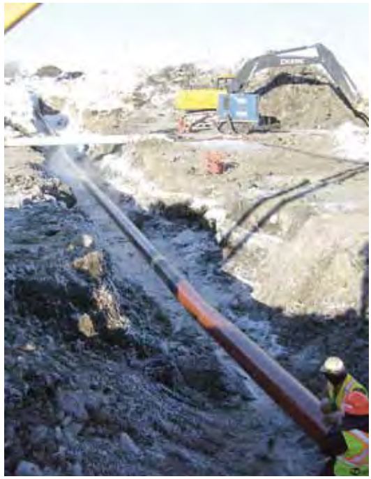
Installation of the 16" natural gas pipeline through the bypass and perpendicular to Sturgeon Creek. The pipe across the trench is the flow of Sturgeon Creek being pumped from upstream to downstream of the dams.
