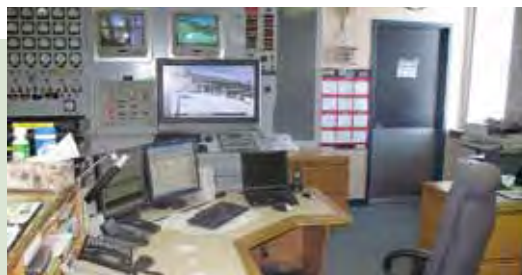
Kettle Control room controlled remotely during off hours has improved the work life balance of employees and is expected to help attract and retain more employees in Gillam and help to reduce operating costs.
