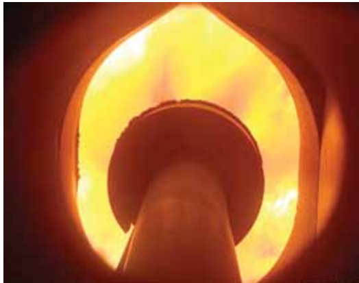
View of burner head as pyrolysis oil is burned in Tolko's Power boiler.
