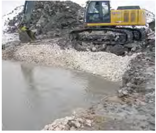
Left: Installation of one of the clay dams ovetop of the clean stone. Right: The downstream Sturgeon Creek bypass dam removed.
