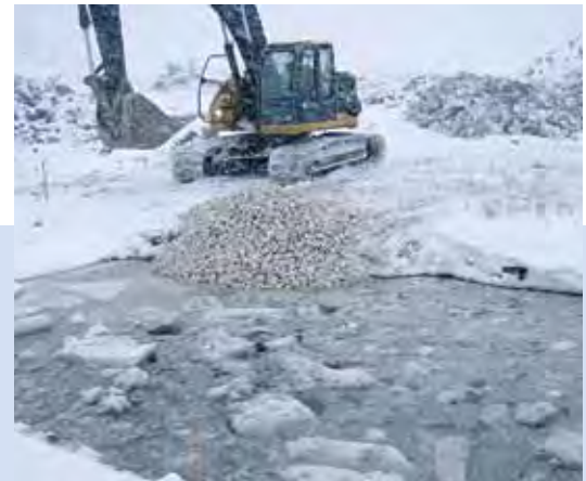
Placing clean stone prior to the clay dams. This prevents downstream turbidity in the water when removing the clay dams.
