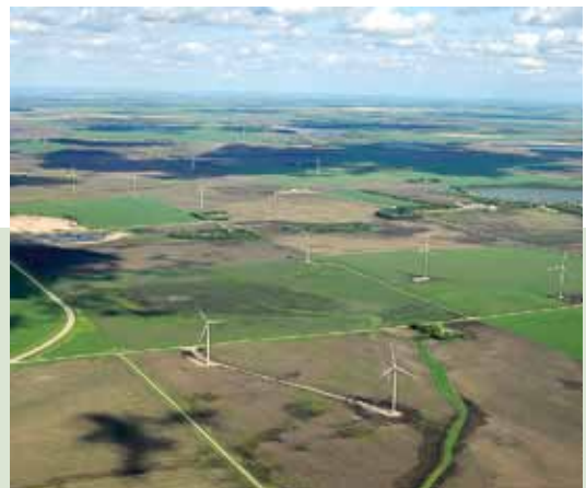
Top: St. Joseph wind farm under construction. Bottom: The wind farm consists of sixty 2.3 MW turbine generators set on 80 m high towers.
